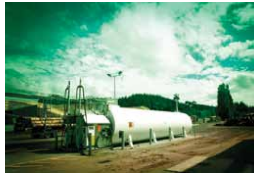
Right, as part of our investment in the Pan Pac business, Greenstone has built a truckstop on a new site with an 80,000 litre diesel tank.
